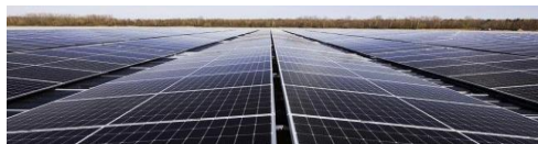
Figure 2. Solar Power Generation
